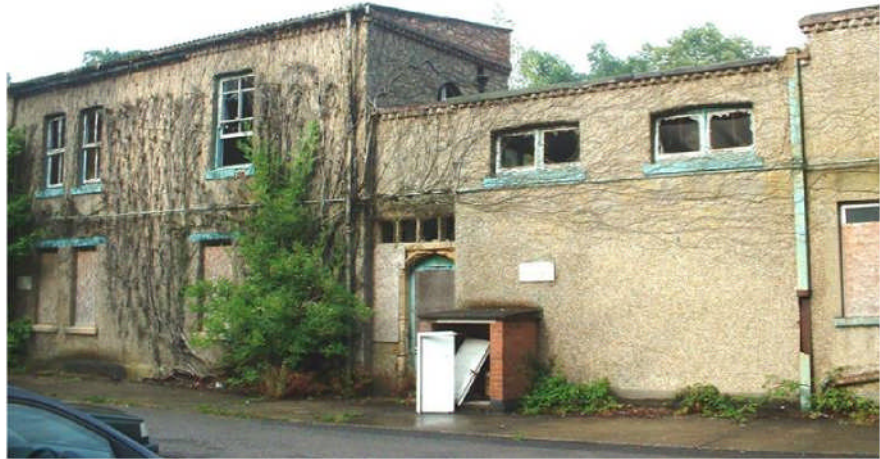
The Derelict Condition of the Spa Baths Today
